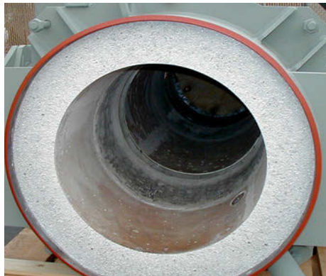
Expansion joint after being thermally dried.
